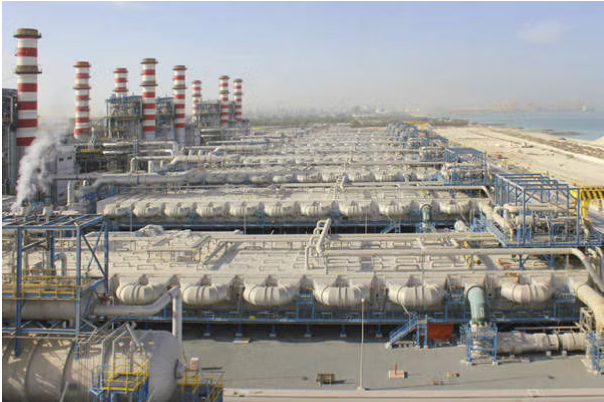
[Jebel Ali desalination plant, Dubai]
